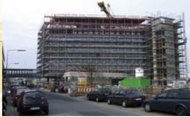
Ten months on: The shell of the building is nearly finished. Part of the glass construction can already be recognized.
