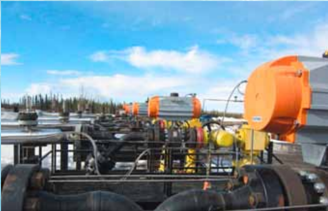
STARLINE ball valves fitted with AIR TORQUE actuators safely control the flow of gas from the well head in the Horn River in northern British Columbia
