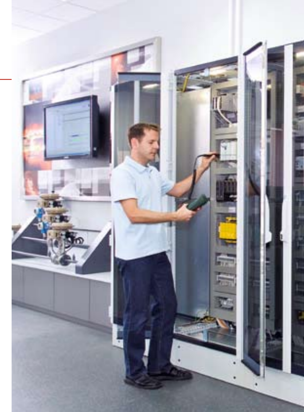
Field components can be integrated into the control systems in the SVIC. While, at the same time, remote access to acyclic diagnosis data is also possible.
