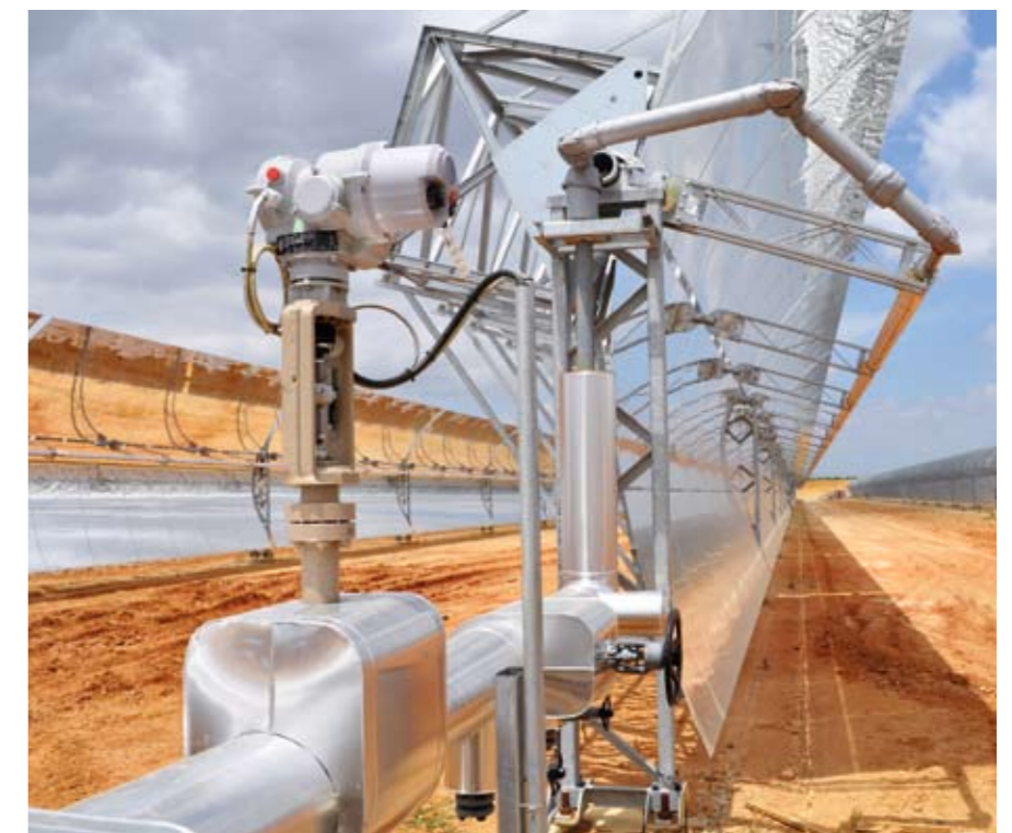
The trough collectors heat the transfer oil up to reach temperatures of 400 °C. 168 Type 3251 Control Valves in NPS 3, Class 600 with bellows and electric actuators ensure optimum flow.
