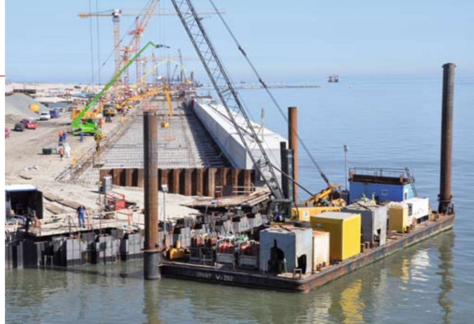
Almost three quarters of all crude oil shipments to Germany arrive at the port of Wilhelmshaven. In anticipation of an expected growth in world trade, a new container port is also being built in the JadeWeserPort.
